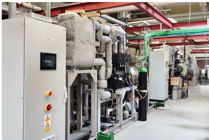
Figure 17: SPH installation in Axilone, Spain for 6 barg steam (source: SPH)
