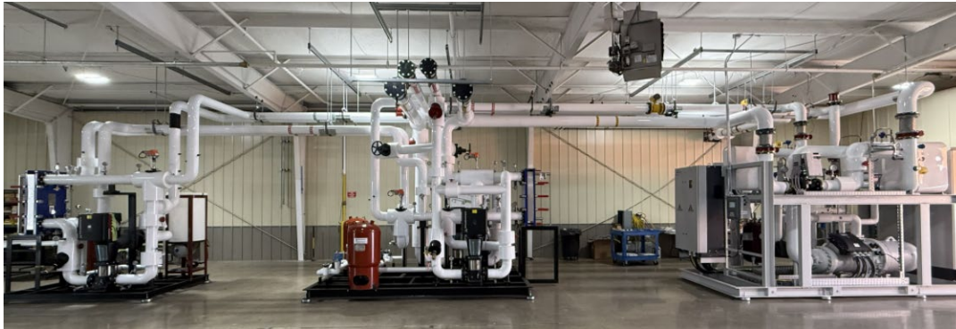
Figure 11: Armstrong IHP in the test facility
