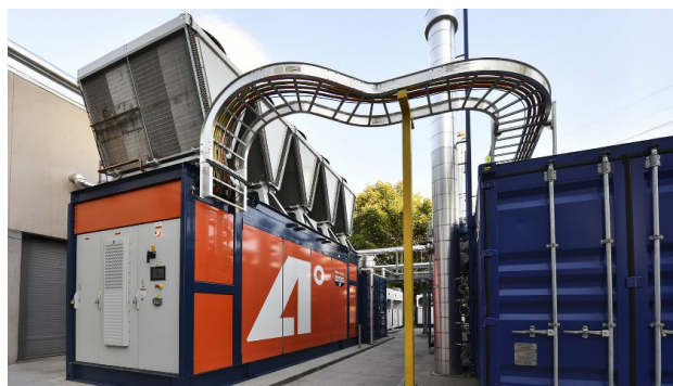
Figure 19: AtmosZero Boiler 2.0 installation at New Belgium Brewery, Ft. Collins, CO
