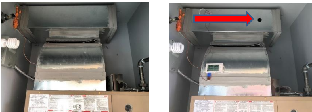
Figure 17: Supply Duct – Left Picture: no hole to weatherize the closet; Right Picture: a small hole to weatherize the closet and mitigate the condensate freezing issues
