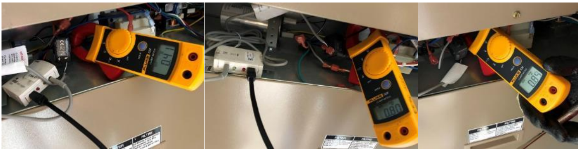
Figure 14: Verification of Fan Motor Current during “On” Call in Apartments 102, 203, and 301
