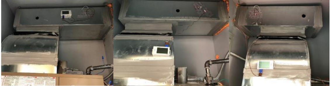
Figure 15: Utility Closet Air Supply Duct Hole, Observed in Apartments 102, 203, and 301 on January 12, 2018
