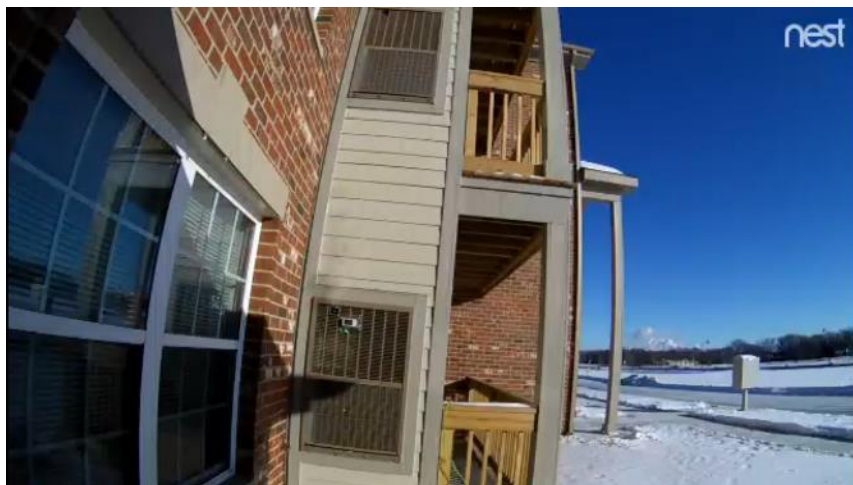
Figure 16: Still-frame from Nest Camera on January 1, 2018 at 14:23:45 Apartment 102 Exhaust visible for comparison with Process Plant Steam in Background
