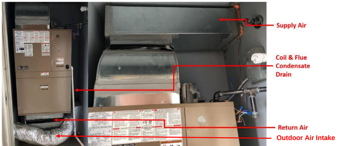
Figure 2: cTTW Furnace/AC Unit in a utility closet
